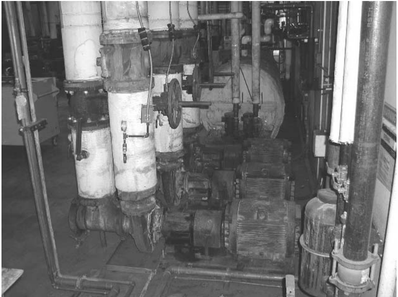
Figure 4-4. Give 50 HP pumps their own equipment number and name.
