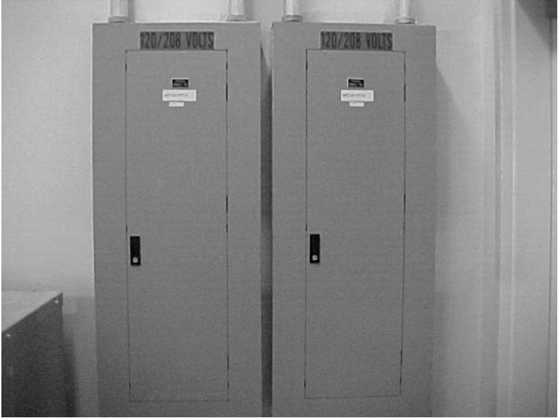
Figure 8-6. Electrical panel on right trips prematurely.
